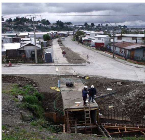
COLECTOR ESTERO LOBOS, PUERTO MONTT
